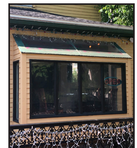
Examples of Incompatible Windows
