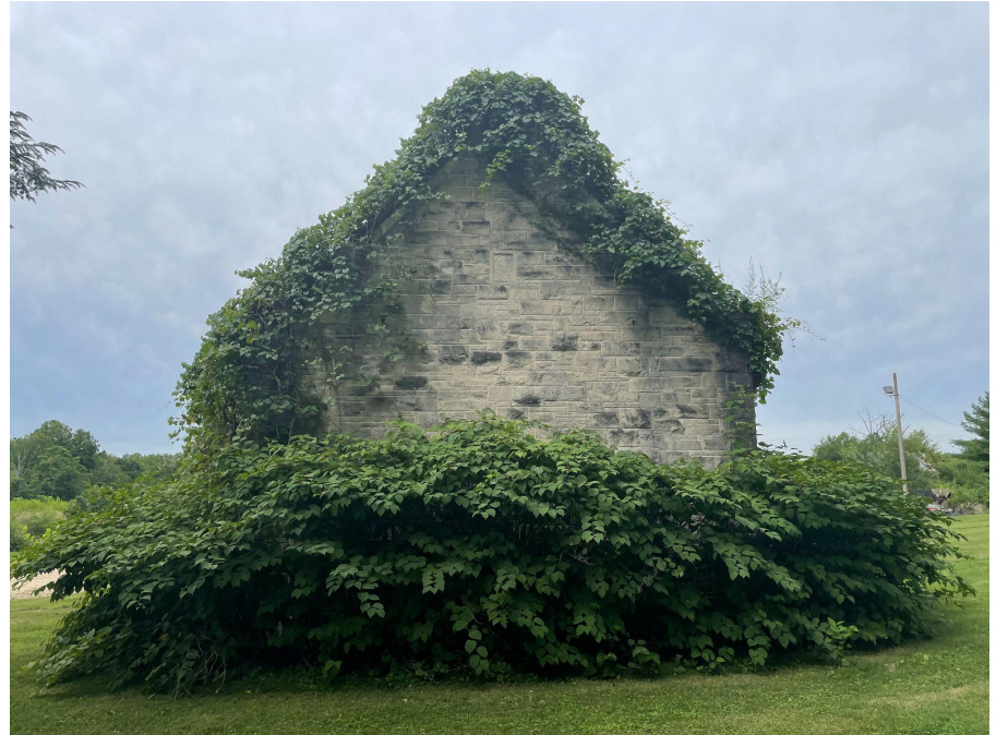
Plans include rehabilitation of limestone building that was the original superintendent house
